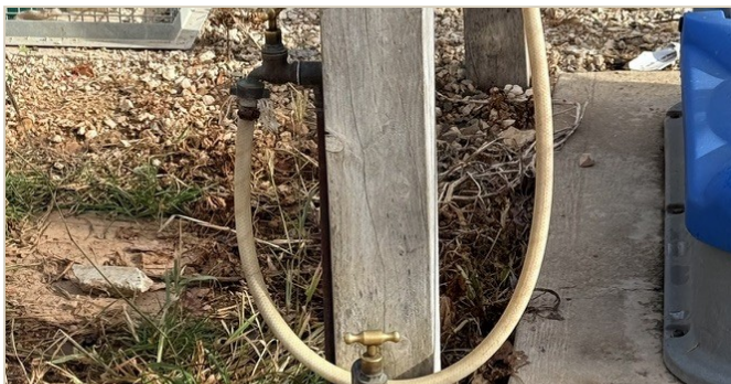
Potable water filling station adjacent to the dump point.
